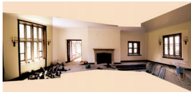
Design Services requested with these jobsite conditions
